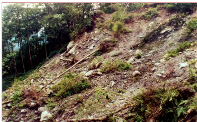
Photo: Slope Failure
