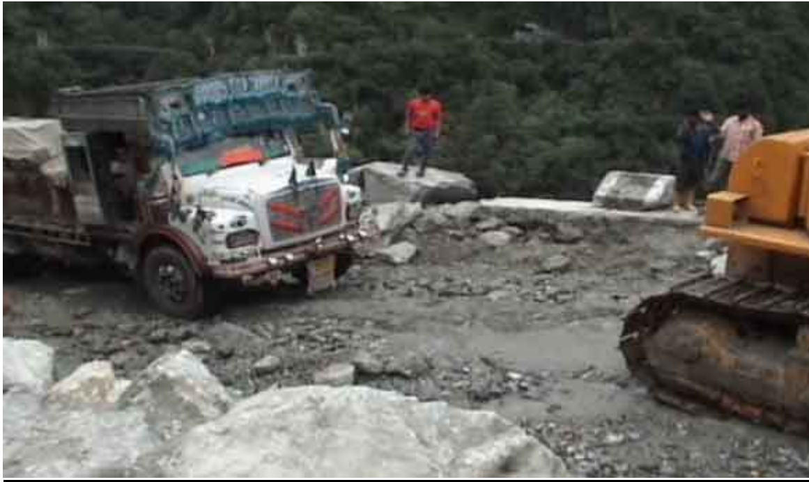
BRO's JCV pulling stuck up loaded lorry in the uphill side at above point.
